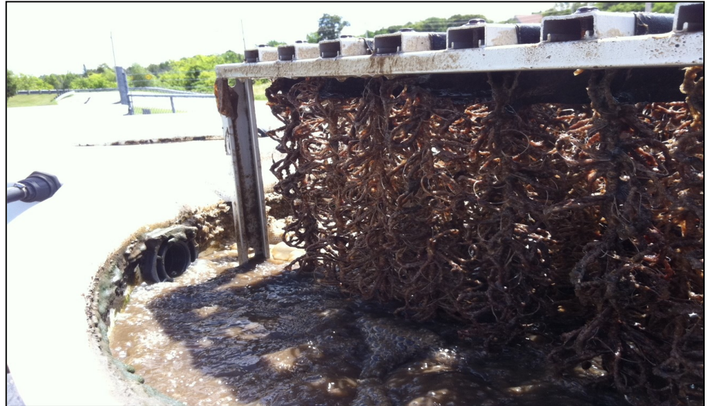
Solid material collected by the Biocord material contained in tank one as it works to biodegrade the sludge
