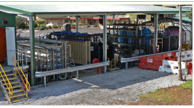
Recycling of treated mine drainage/discharge water for process and potable purpose within coal mining industry, Australia
